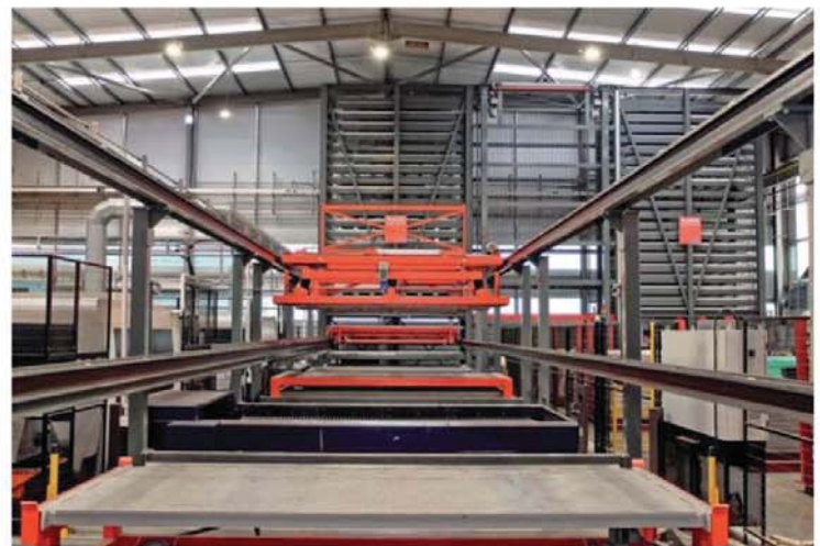
Another view of the automated storage system showing the handling arrangement serving the two other fibre laser machines
